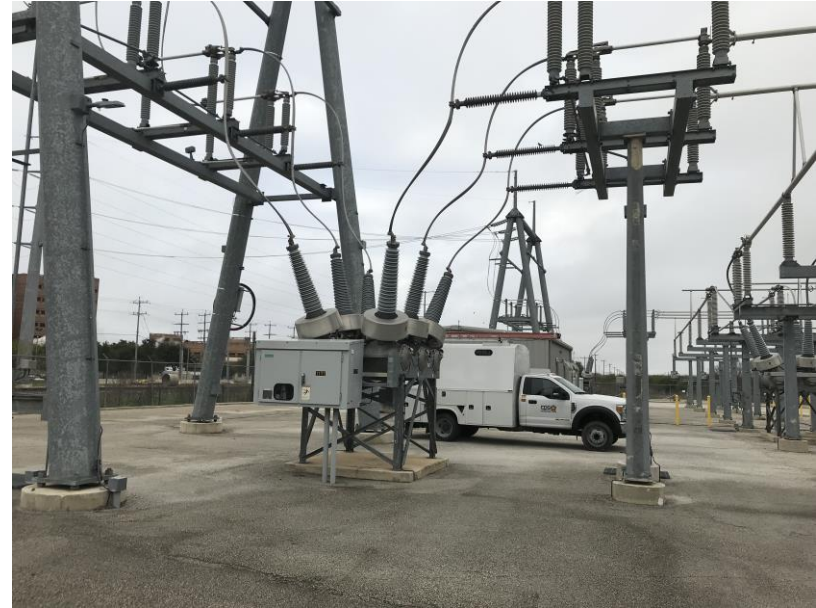
138kV Breaker Number of Breakers: 561 Purchase Price/Breaker: $78K
