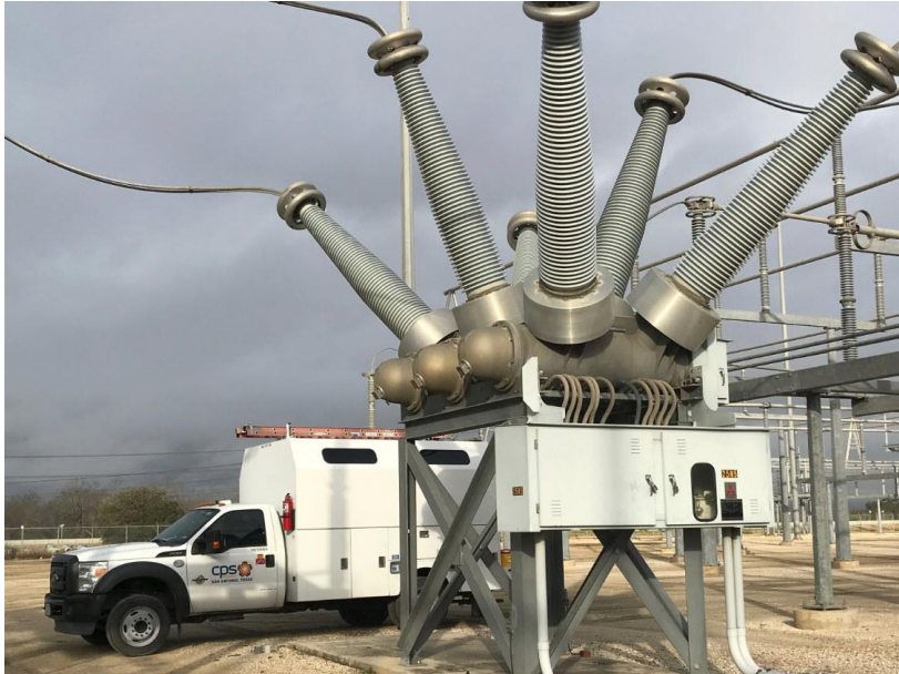
345kV Breaker Number of Breakers: 80 Purchase Price/Breaker: $210K
