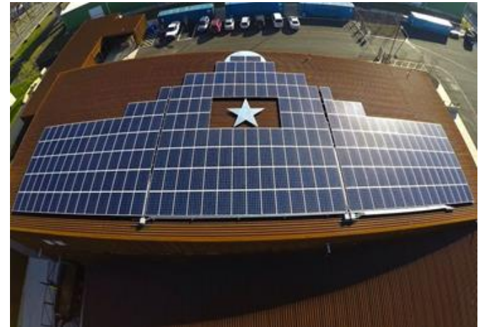
Rooftop solar installation at Alamo Beer Company
