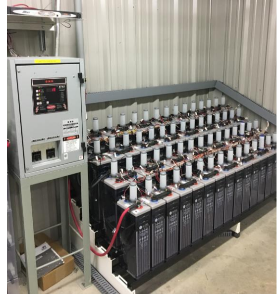
Installed battery monitoring system – partially automated
