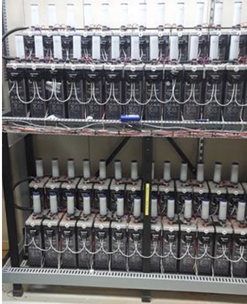
Installed battery monitoring system – fully automated
