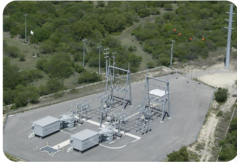
Hamilton Wolfe Substation
